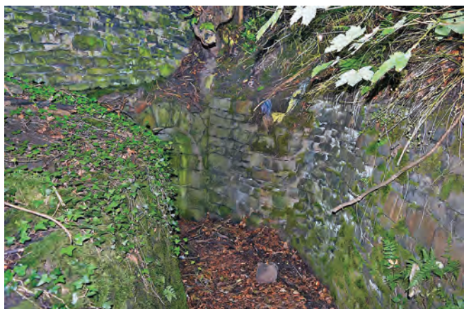
The north entrance to the subway showing 90 degree turn from the approach path to the tunnel itself
